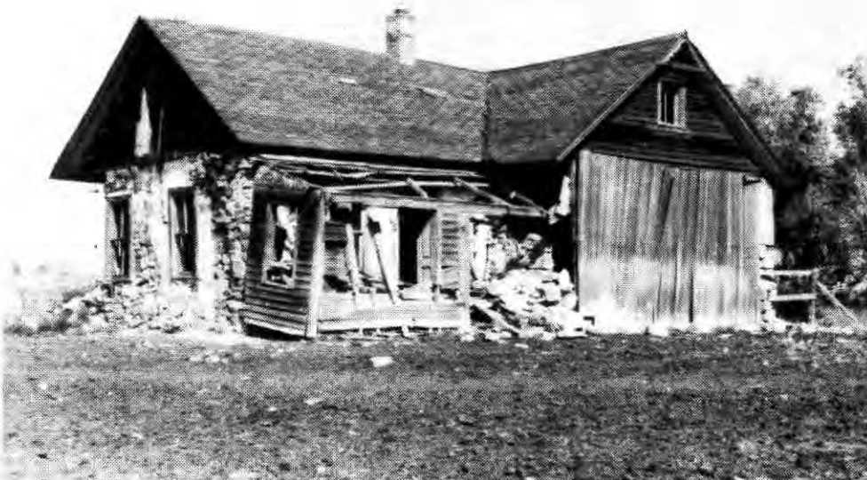
Figure 28. Froehlich House [32 SK 181] showing large kitchen addition to the facade.
