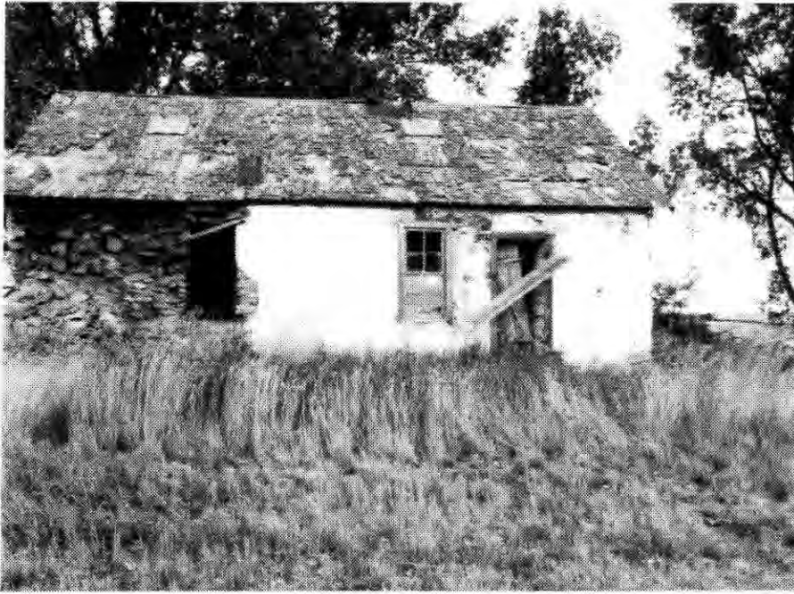
Figure 13. Two-room house at Joseph Kuhn Farmstead [32 SK 187]. Wall on left is partially collapsed exposing stone.
